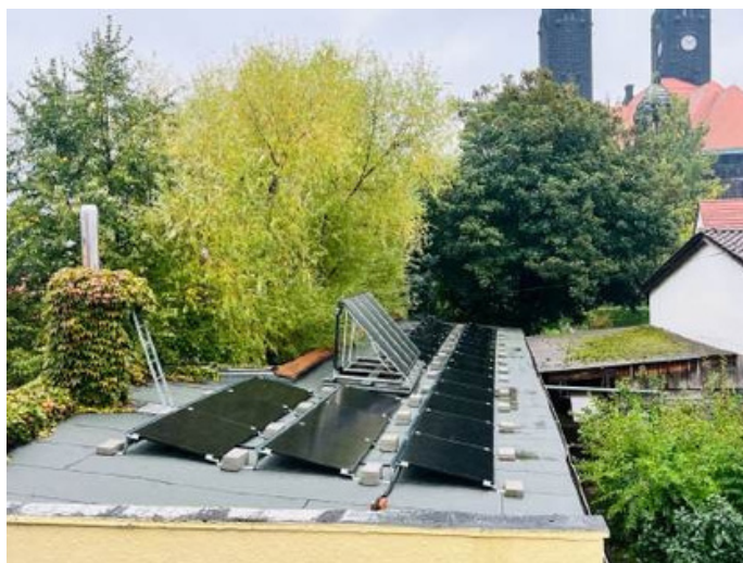
AS Photovoltaik & Solarthermieanlage
